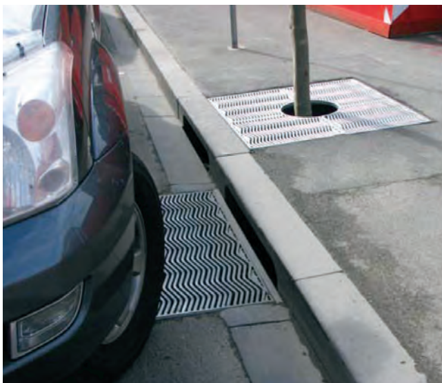
Fig 10a Typical design of a raingarden street tree with customised grate and overflow grate located along the kerb.
