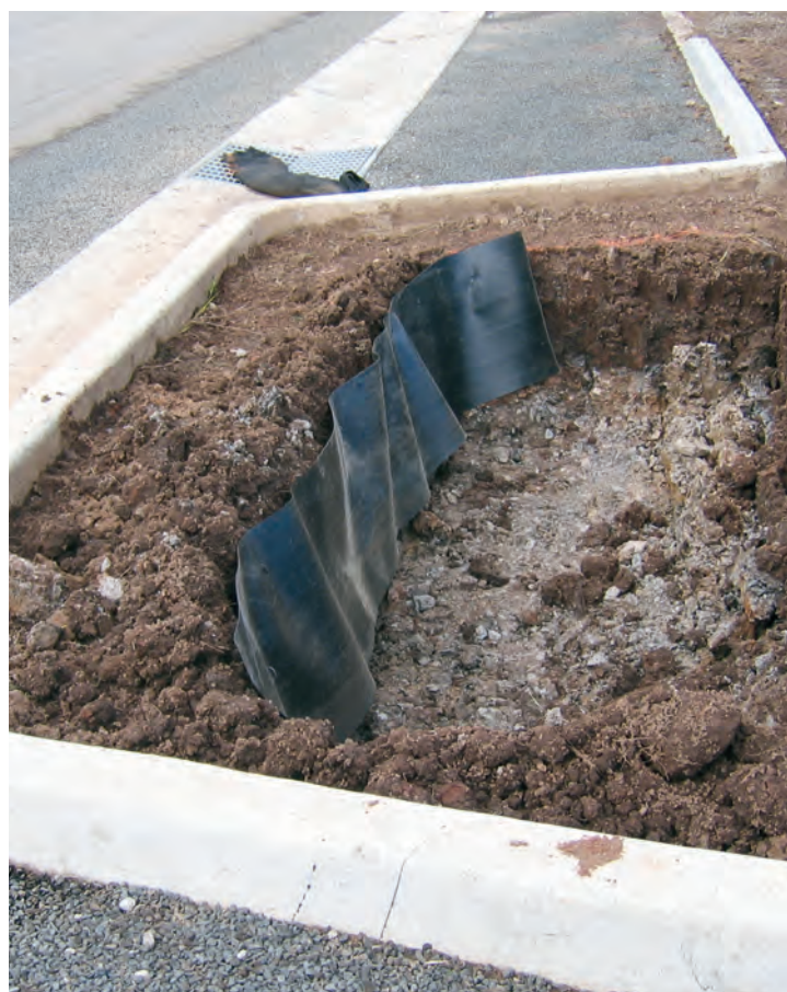
Root barriers installed to protect public utility and road assets however a better solution is providing trees with adequate soil volume.
